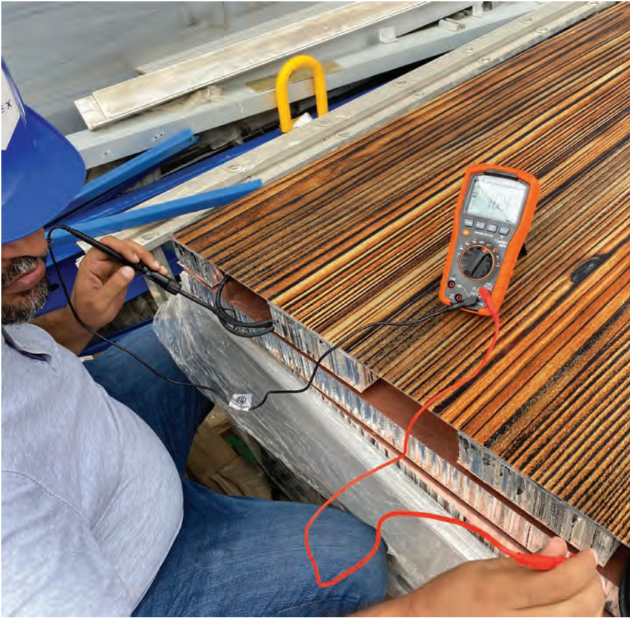
Testing Voc of Facade Solar Panels
