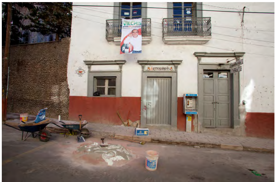
There always seemed to be a lot of repair and construction work under way.
