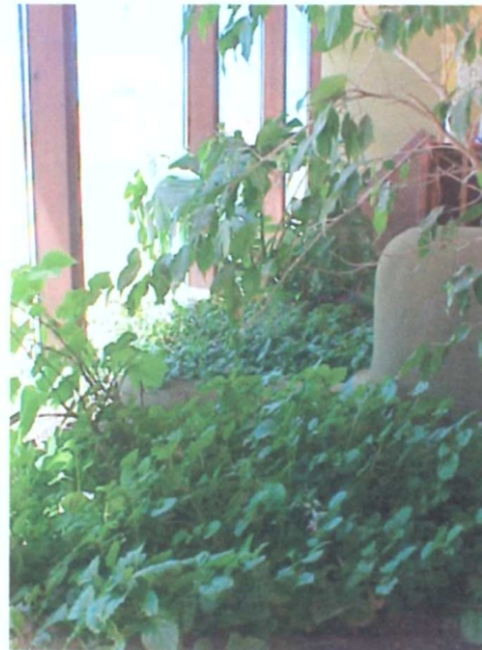
Gray water treatment planter
