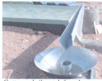
Gutter and silt catch funnel
