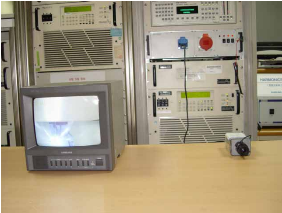
Picture 5. Harmonics & Flicker
